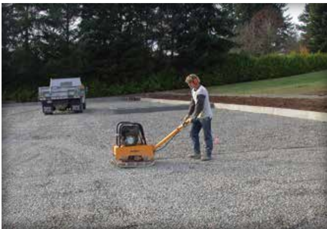
Figure 21. A 13,500 (60 kN) vibratory plate compactor is used on this ASTM No. 57 stone base.
